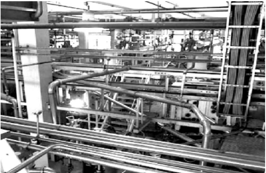
FIGURE 8. Example of inappropriate piping.
